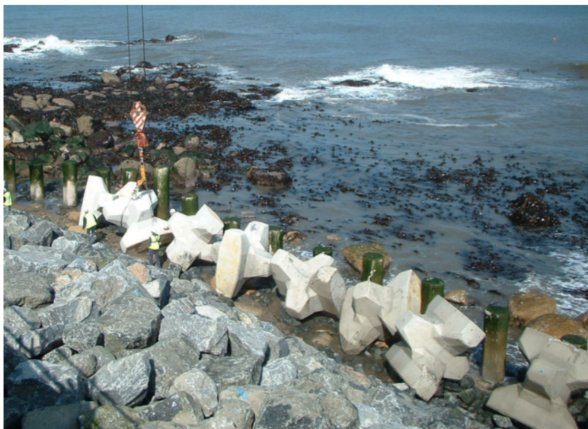
Figure 9: Placing the first row of Accropodes™ against a toe structure of concrete piles (Scarborough, UK)
