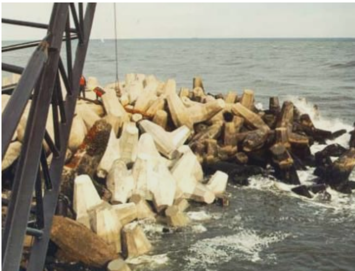
Figure 5: Repair of Dolos armouring with Core-loc® (Jetties at Manasquan Inlet, New Jersey, USA)
