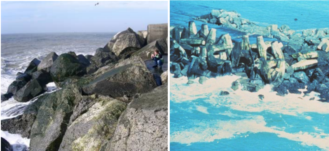
Figure 3: Breakage of armour units: Cubes (left) and Dolos (right)
